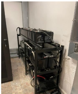
Paneli i UPS
