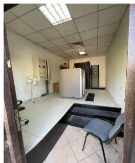
Paneli i UPS
